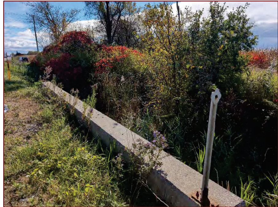
Image 36: County Road 46 – Gas Facility
