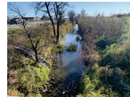
Watercourse Crossing 9 runs parallel to County Road 19 and is conveyed under County Road 46.
