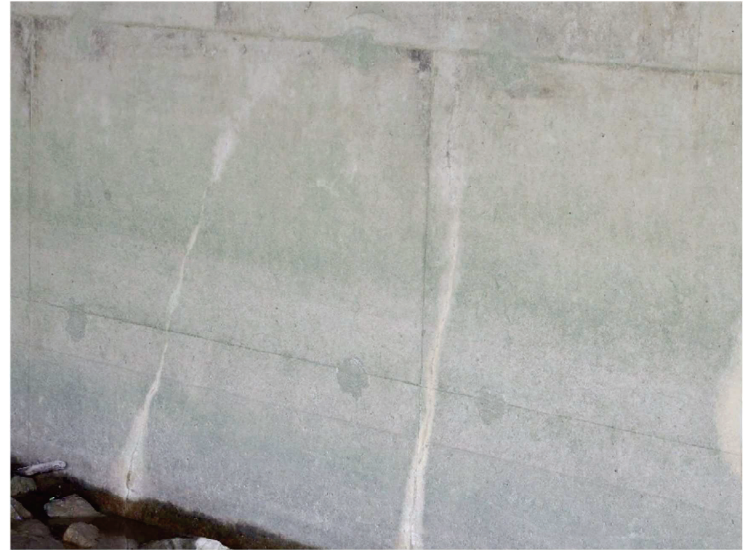
Figure 7 - Narrow Cracking on East Abutment Wall
