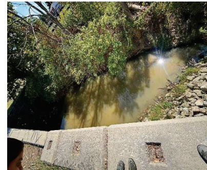
Photo 36: Pooled water at culvert inlet at Crossing 7, south side of County Road 46.
