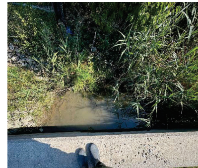
Photo 17: Pooled water at culvert outlet of Crossing 4, north side of County Road 46.
