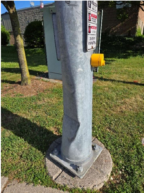
Figure 33: Traffic Signal Pole
