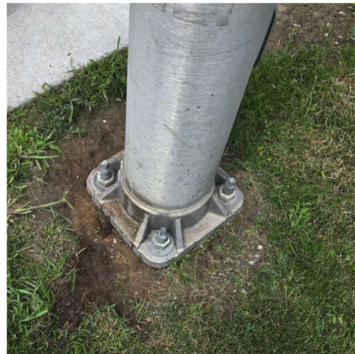
Figure 41: Traffic Pole Base
