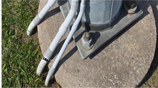
Figure 25: Power Supply Conduit
