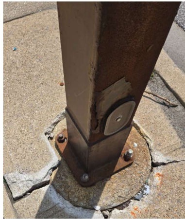
Figure 9: Painted Pole with Peeling Paint
