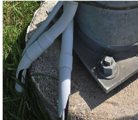
Figure 20: Power Supply Conduits
