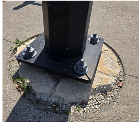
Figure 16: Concrete Spalling and Peeling Paint
