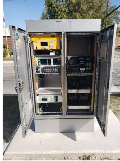
Figure 11: New Cabinet and Controller
