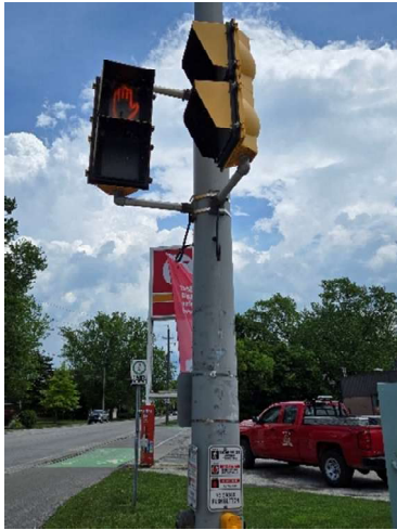
Figure 4: Painted Pole with Peeling Paint
