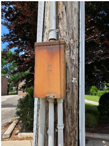
Figure 2: Power Supply Cabinet
