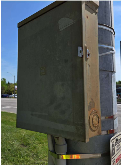
Figure 19: Power Supply Cabinet
