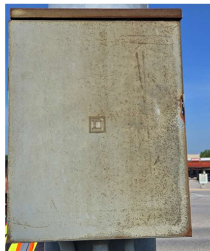
Figure 24: Power Supply Cabinet
