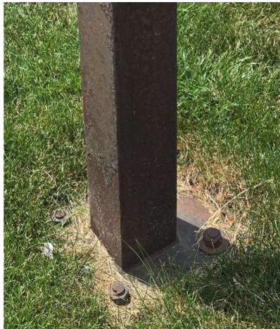
Figure 8: Painted Pole with Peeling Paint
