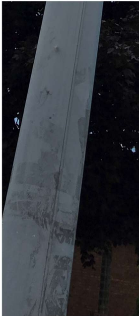
Figure 5: Painted Pole with Peeling Paint
