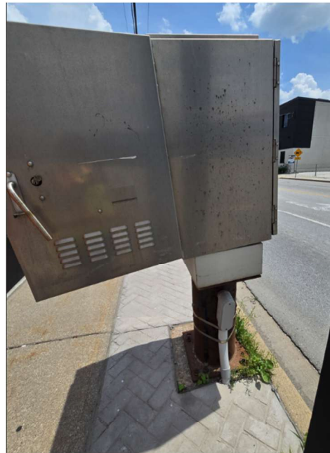
Figure 39: Traffic Signal Cabinet
