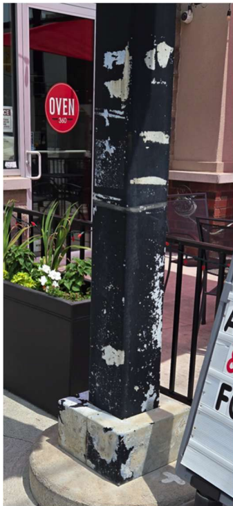
Figure 38: Painted Pole with Peeling Paint
