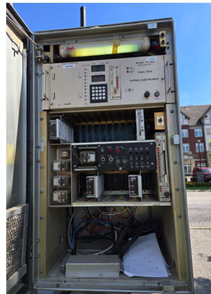
Figure 18: Pole Mounted Cabinet with 170 Controller
