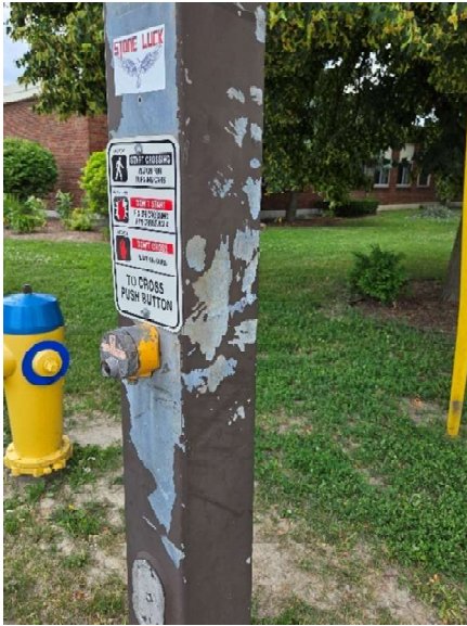
Figure 10: Peeling Paint and Push Button
